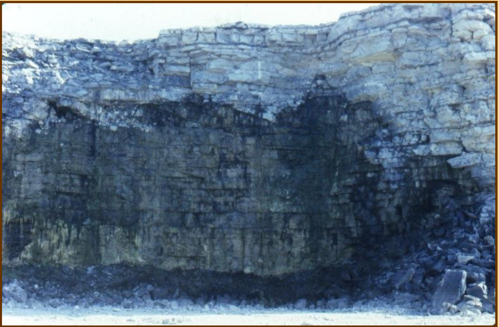
Seepage on Highwall Face
