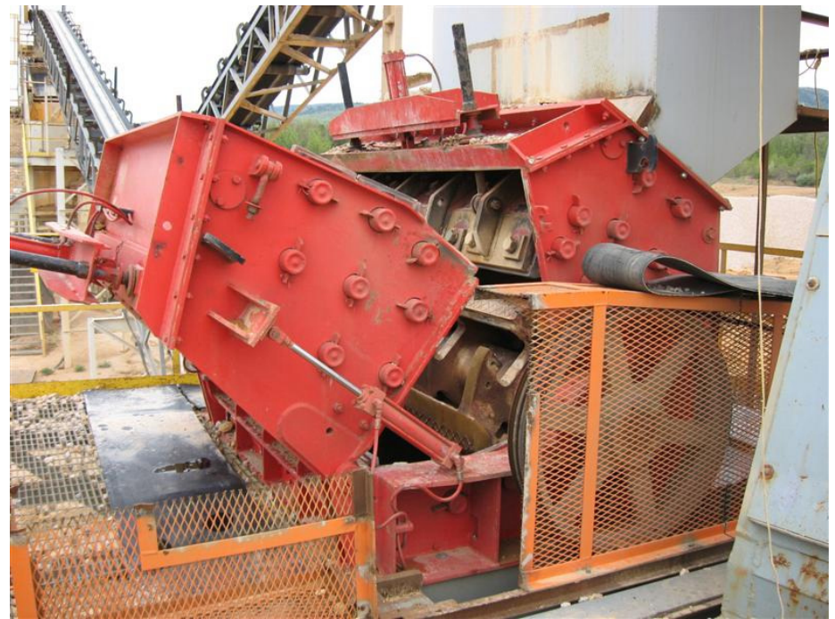
Impact crusher involved in accident
