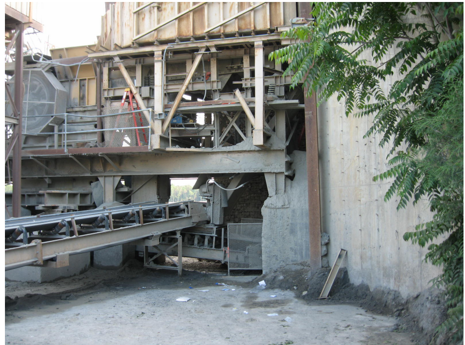
Miner fell from platform in top center of photograph
