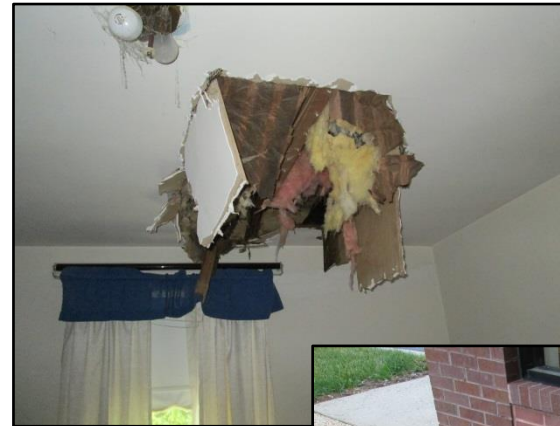
Ceiling damage at home where occupant was injured.
