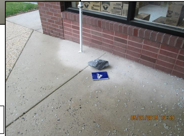
Rock that damaged a storefront.
