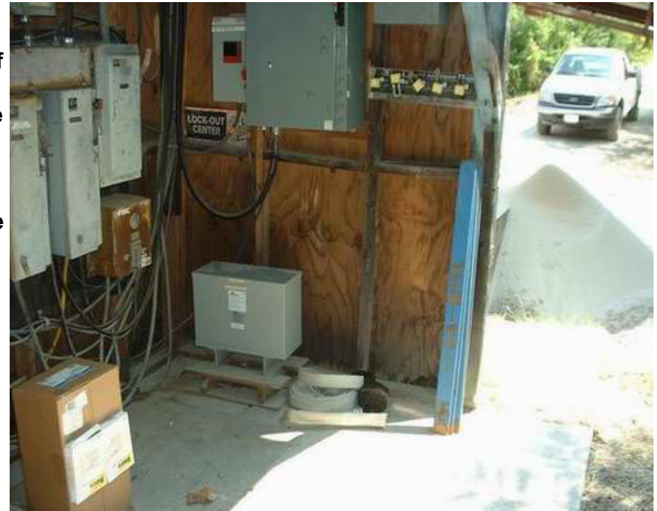
Barge load-out building where snake-bite occurred. Note rolled up fire hose on floor where snake is thought to have been located.
