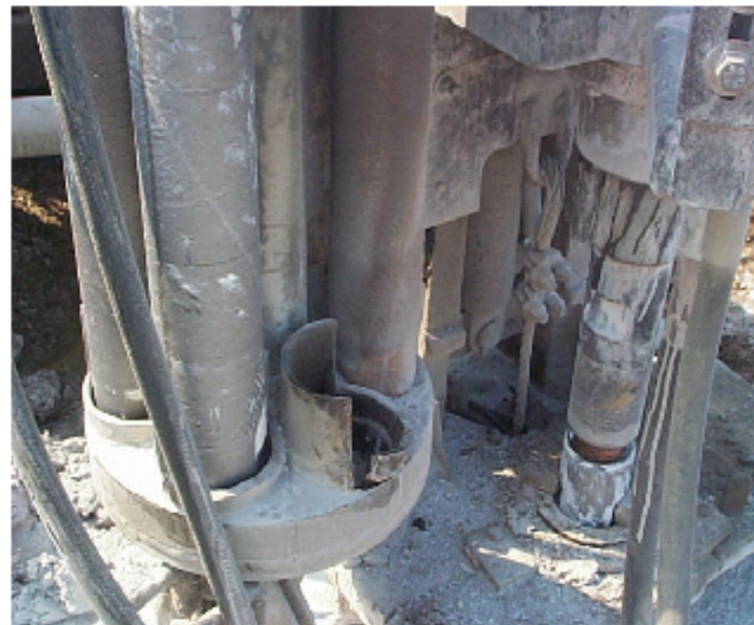
Steel rods in the carousel are held in place by a spider hook on top, and a pod (cup) on the bottom; pod bent outward when rod fell out of the carousel.
