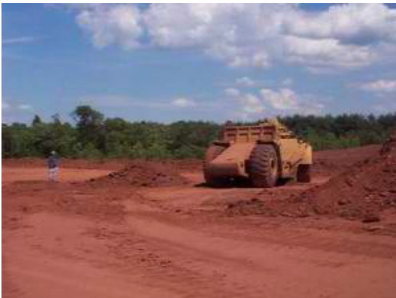
The scraper after righting. Note small pile of material that was dumped when the scraper turned over.
