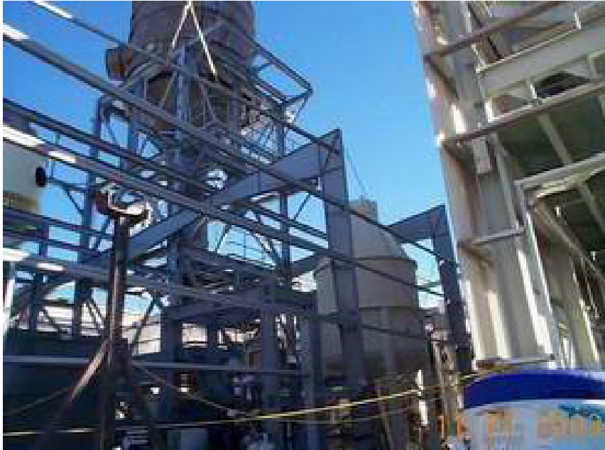
Victim was sitting on the large structural steel beam shown in center of photograph prior to fall.
