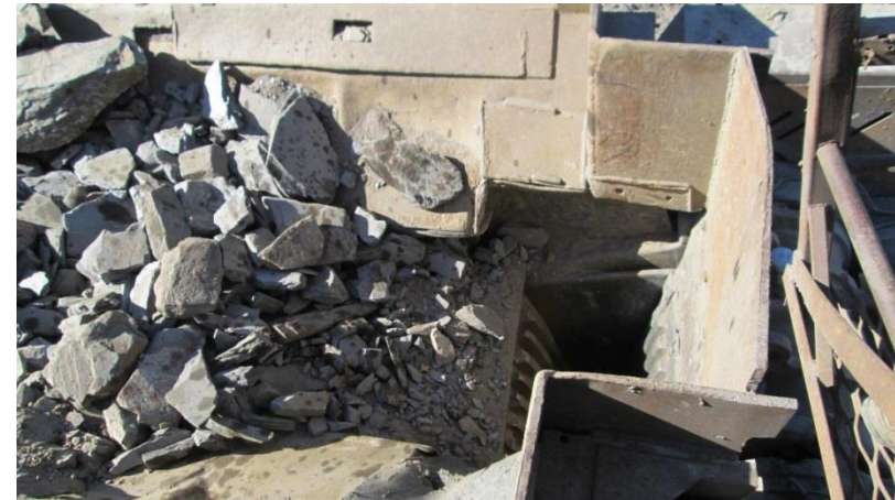
Feeder and crusher opening where accident took place
