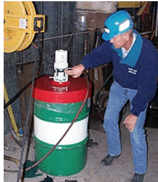
The Graco pneumatically powered grease dispenser pump without required guards (cover plates) in place.
