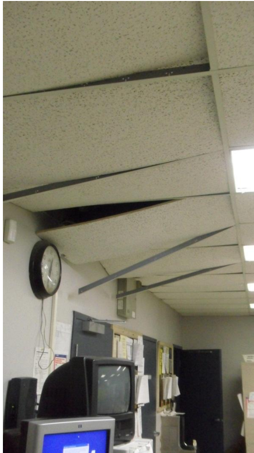
Figure 49. Ceiling tiles that fell along the North wall in the Mineral Post Office (38.00669, -77.90859).
