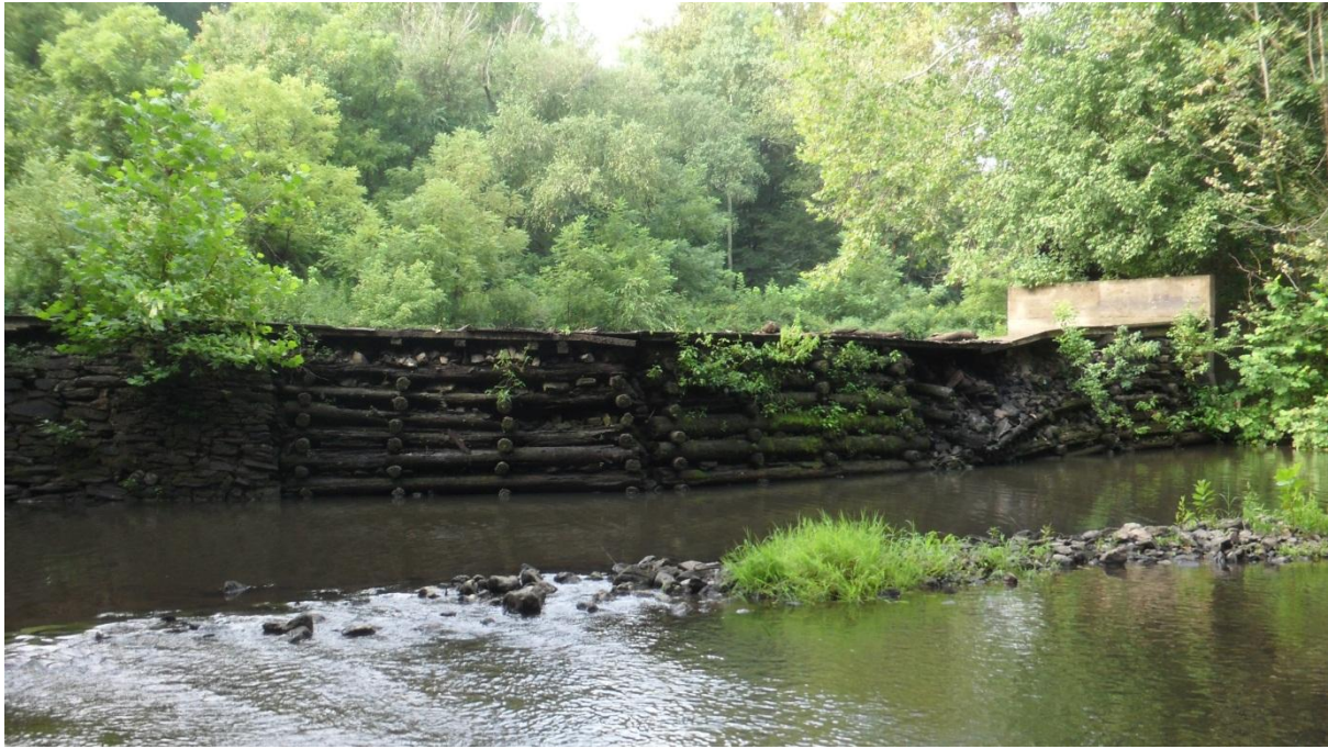
Figure 33. Yancy Mill Dam. It is unknown whether the damage shown in this photo resulted from the earthquake, but the owner was not aware of any pre-earthquake damage to the dam (37.93825, -77.98300).
