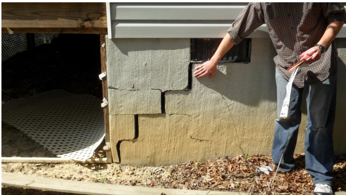
Figure 51. Typical damage to block foundation walls (37.9790, -77.9692).
