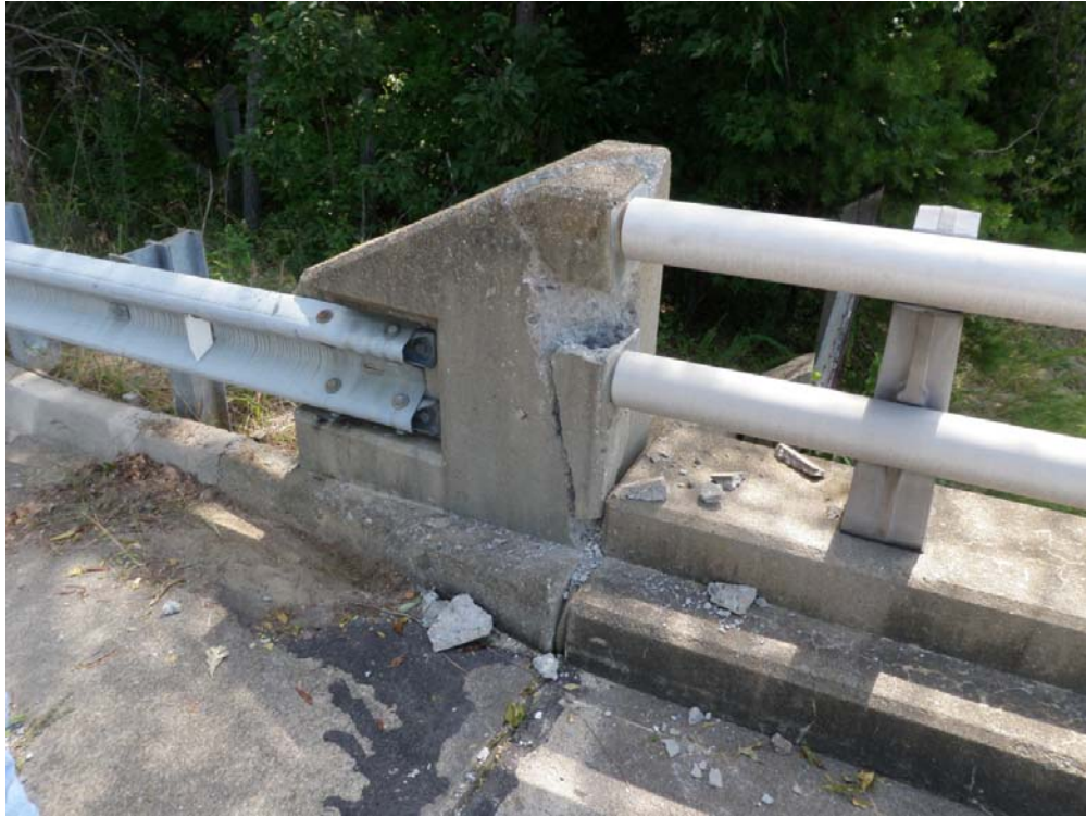
Figure 5-5 Parish Road over Interstate I-64 –spalling (37.89477, -78.04297).
