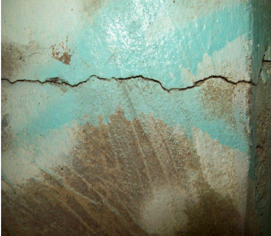
Figure 5-7 Route 1 over Hazel Run – horizontal crack at Column 3, Pier 1.
