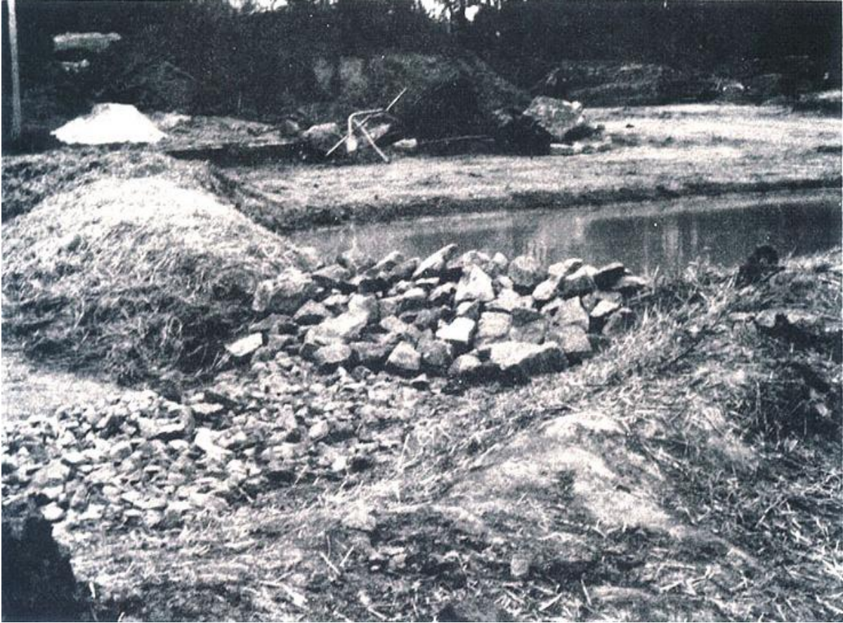
FIGURE 7. Example of temporary sediment trap
